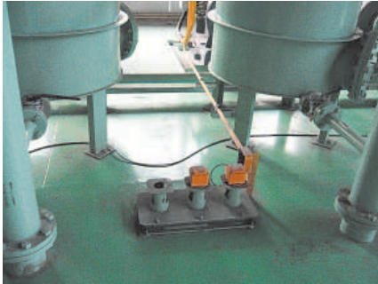
Level sensor attached to prevent overflow of the circulating water pit (Eco Technologies Company)
