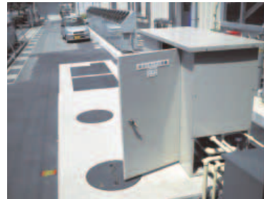
Discharged water recycling device (Subaru Fukuoka PDI Center)
