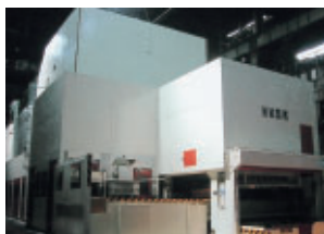
Stamping press equipped with sound insulation (the Second Stamping Section, Yajima Plant, Gunma Manufacturing Div.)
