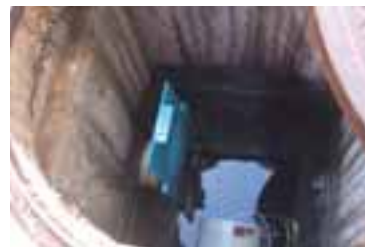
A cut-off valve based on an employee's idea placed on the oily water separating tank
