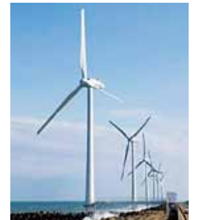
The SUBARU 80/2.0 wind-power generator system
