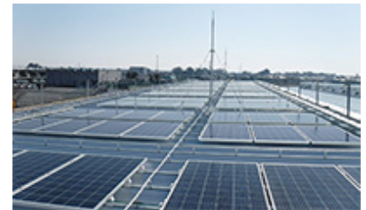
Oizumi Plant of Fuji Machinery Co., Ltd.
