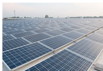
1 MW Power Generation Facility
