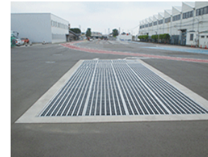
Flood prevention measure (drainage grid) (Utsunomiya Plant)
